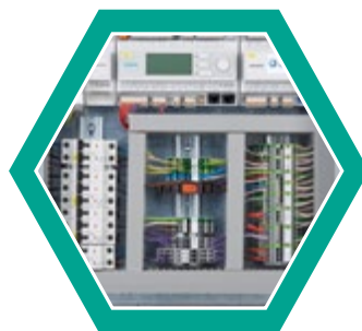
High quality standards for wiring
